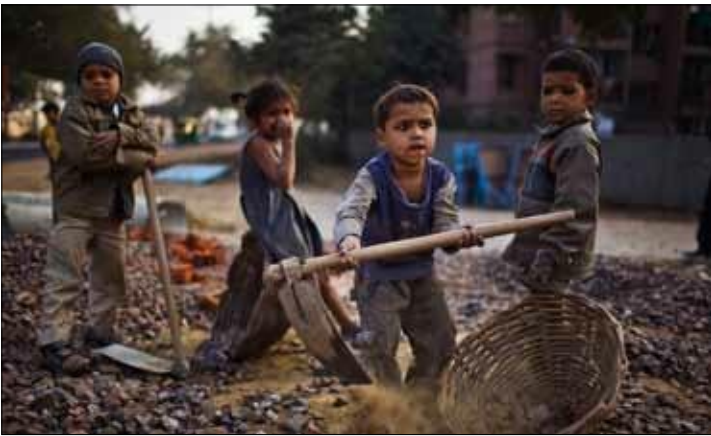
Indian children work at a construction site in New Delhi, India. The construction project is one of many aimed at enhancing the city's sporting and transport infrastructure in advance of the October 2010 Commonwealth Games. Migrant workers from all over India are being paid below the minimum wage and are living and working in substandard conditions to complete these projects.
